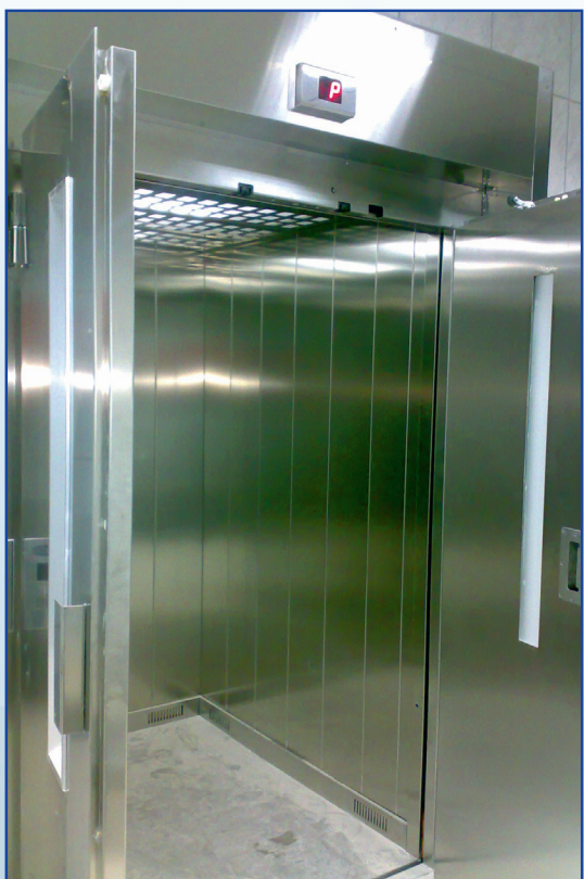
Zidovi inox, pod guma, strop inox Inox walls, Rubber floor, Inox ceiling Wände Inox, Fussboden Gummi, Decke Inox
