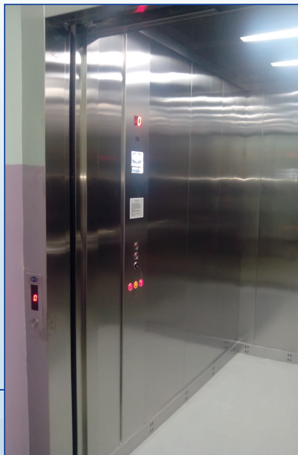
Zidovi inox, pod guma, strop inox Inox walls, Rubber floor, Inox ceiling Wände Inox, Fussboden Gummi, Decke Inox
