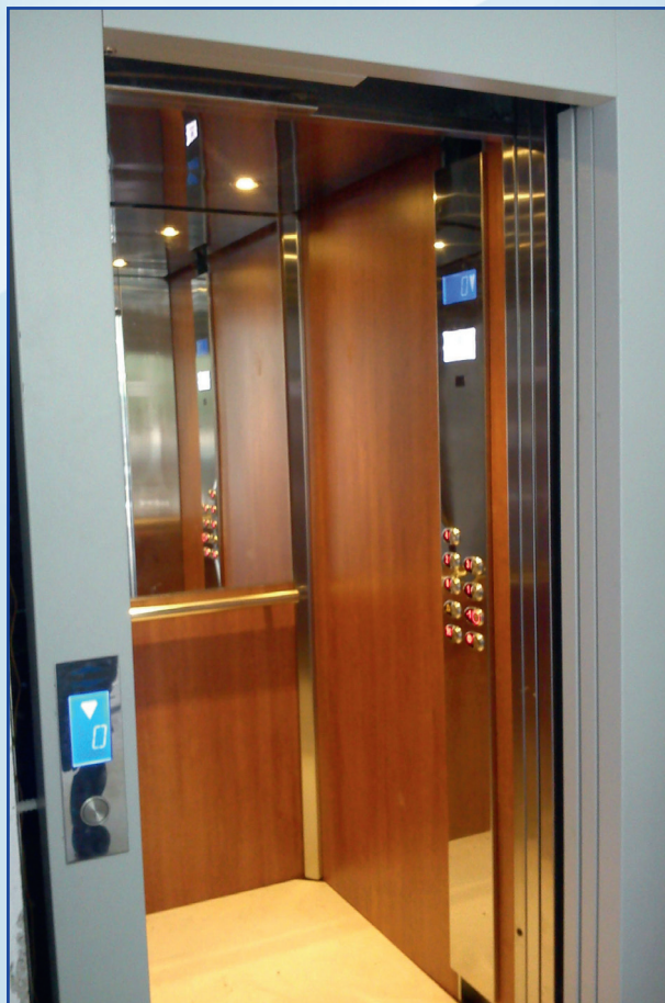
Zidovi laminat, pod guma, strop inox Laminate walls, Floor Rubber, Inox ceiling Wände Laminat, Fussboden Gummi, Decke Inox
